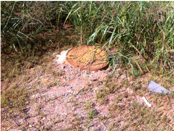
This area contains deteriorating infrastructure.
