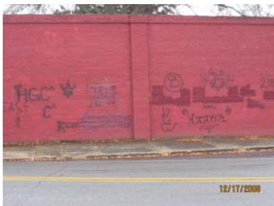
This area contains sections of neglect.
