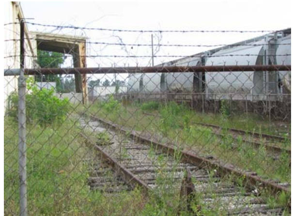
This area contains deteriorating rail spurs.
