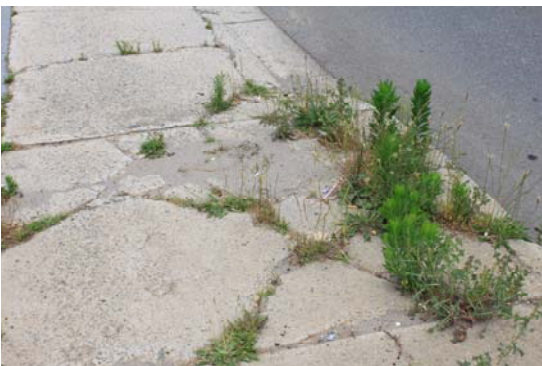
This area contains deteriorating infrastructure.
