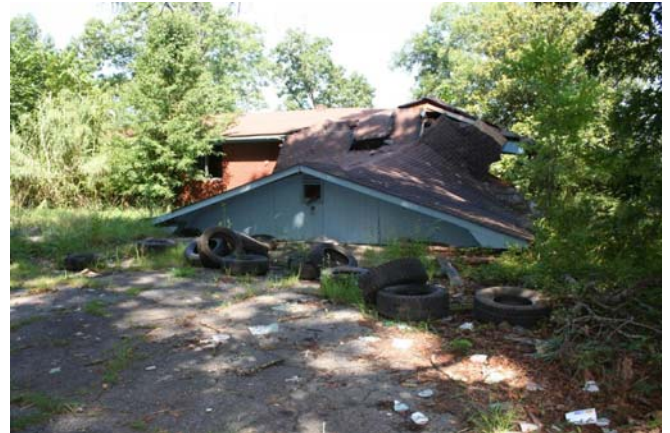
Collapsed structure on vacant lot, Carson Loop
