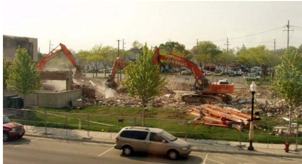
The former 1966 downtown Aurora, Illinois police station was demolished and will be a park.
