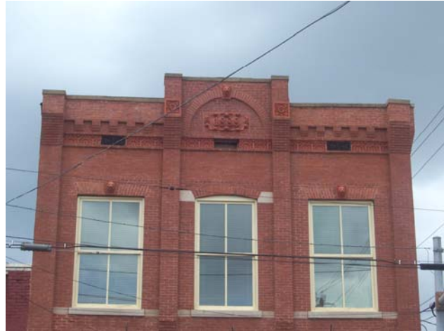
Image 2: The Stein Building, Main St. The original cornice has been well maintained
