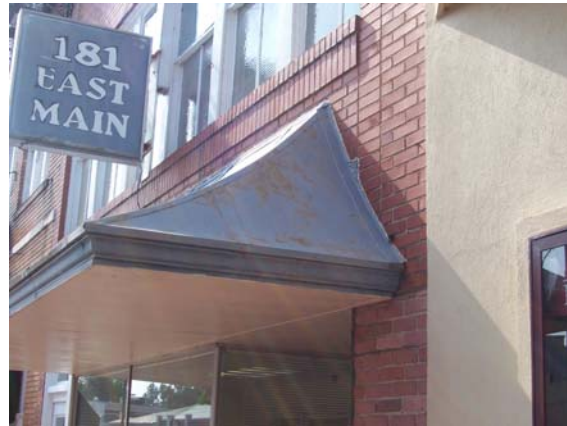
This rusted metal canopy needs replacement
