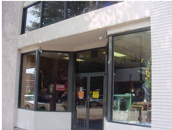
The original windows have been replaced by ones that do not match the historical area.
