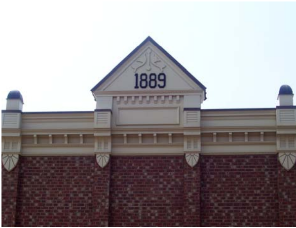
Image 1: Knight's Building, Main St. A new cornice has been reconstructed from historic pictures
