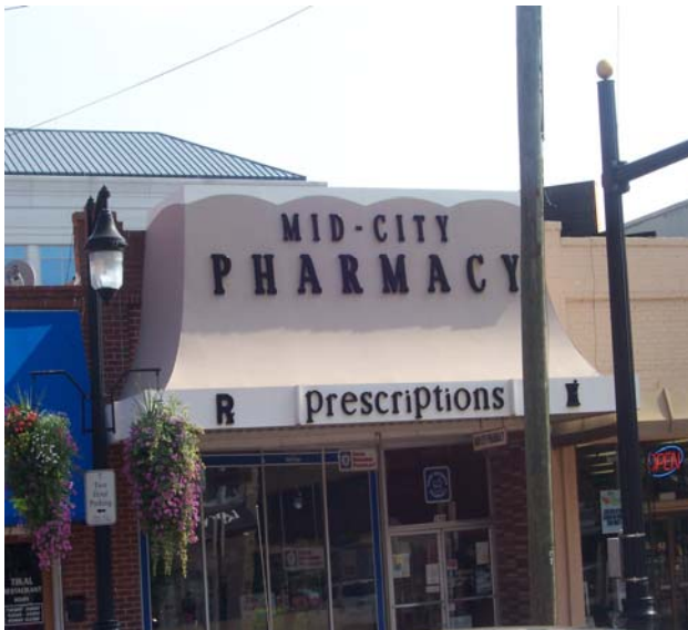
In this example the original cornice is covered by a large sign.
