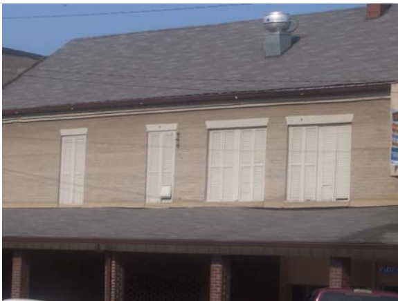
It is not appropriate to block fill in windows
